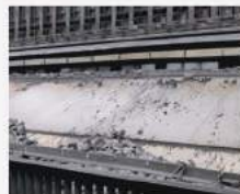
Liner plates in coke plant cooling bed
